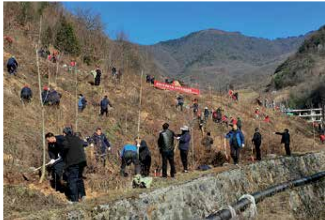
Planting native trees and stabilizing a slope in Shennongjia UNESCO Global Geopark.
