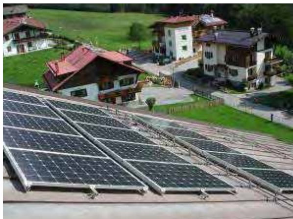
Fig. 1: Photovoltaic panels – guest house S. Antonio di Mavignola
